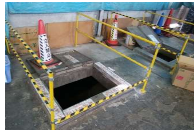
Safety measures for waste storage sites
